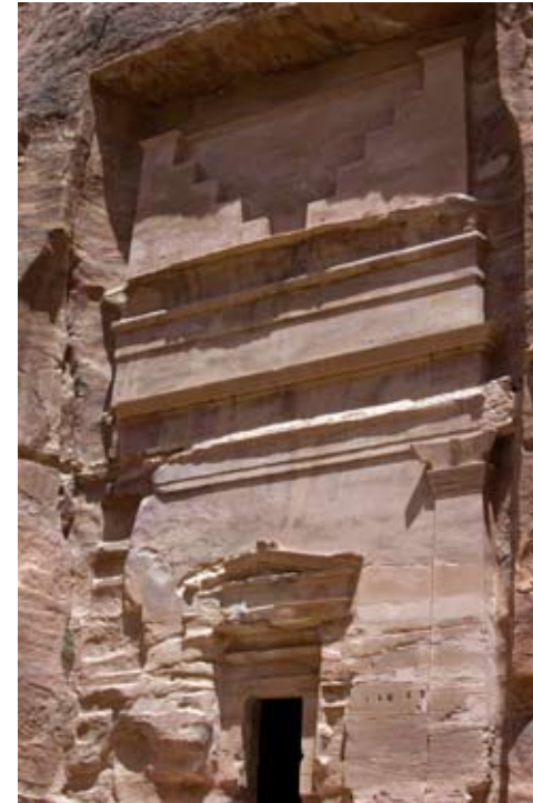
FAÇADE IN SLIGHT DISREPAIR
