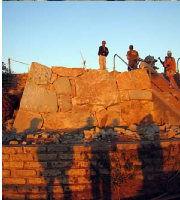
TOP: FINISHING OUT THE SECOND RAMPART. BOTTOM: SOME WORK DAYS RAN LONG.
