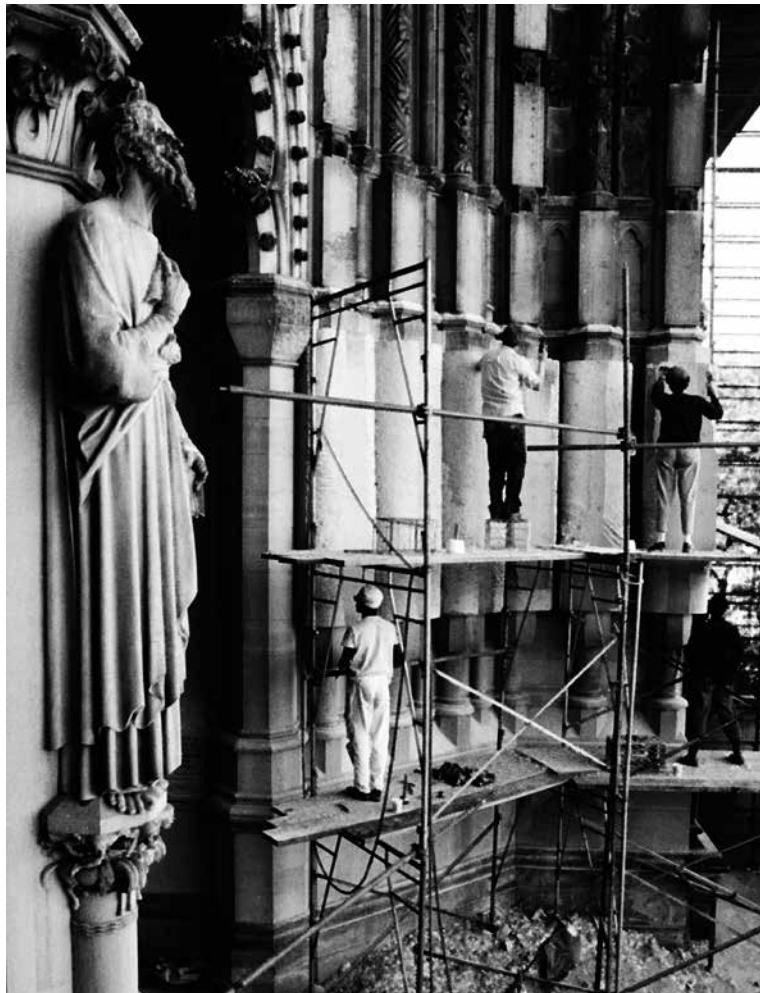
▲ ROUGHING OUT STATUE BLOCKS (PLACED IN 1920'S) OF CATHEDRAL CENTRAL PORTAL, 1988. PHOTO: ROBERT RODRIGUEZ
